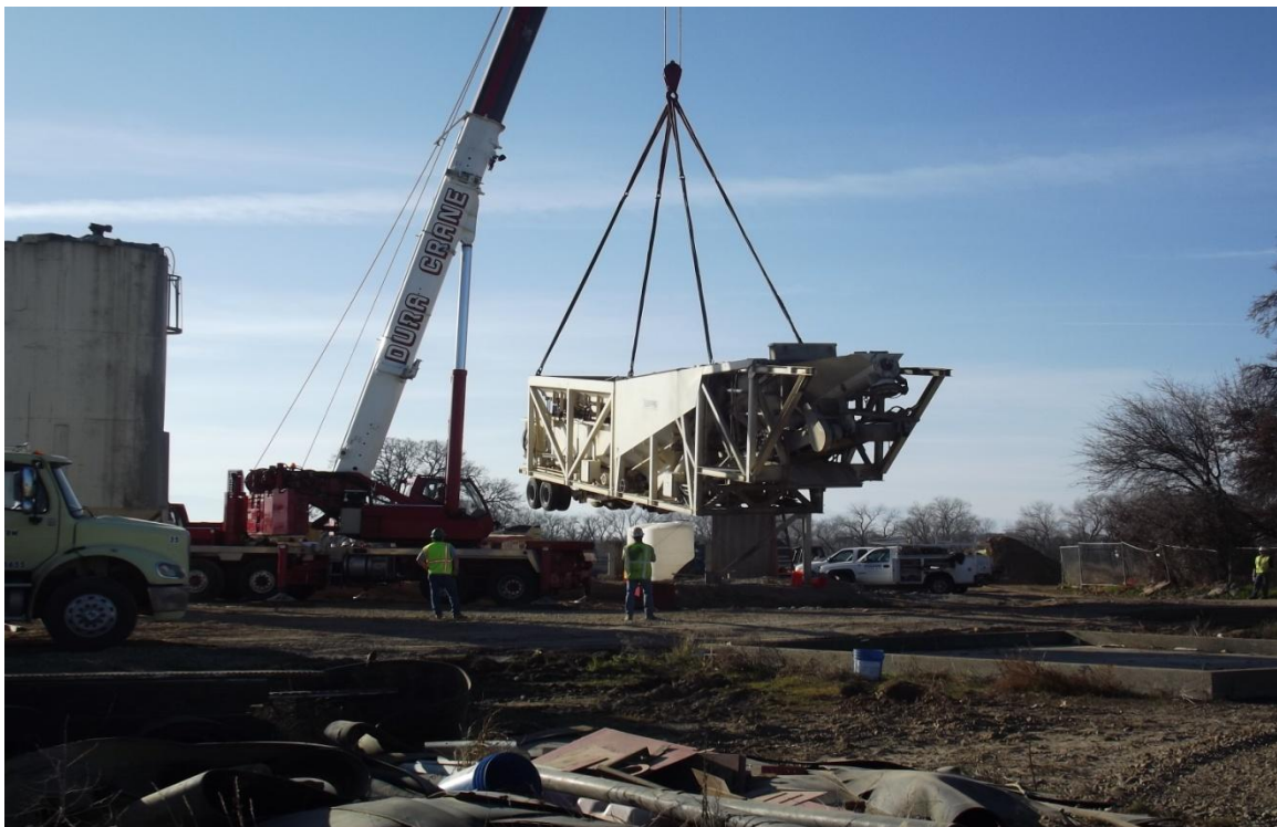
West Bay Builders subcontractor Dura Crane assisting Folsom to rig batch plant platform.
