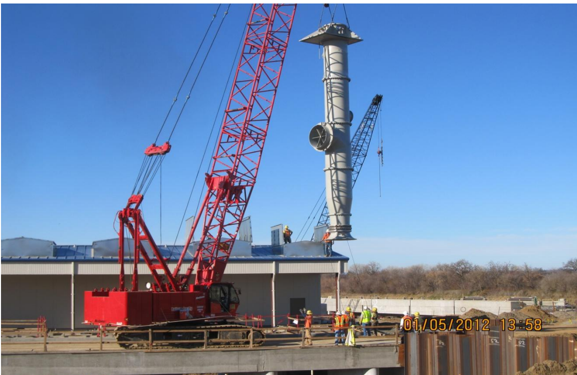
Balfour Beatty installing 60" diameter pump through Pumping Plant control building roof hatch.
