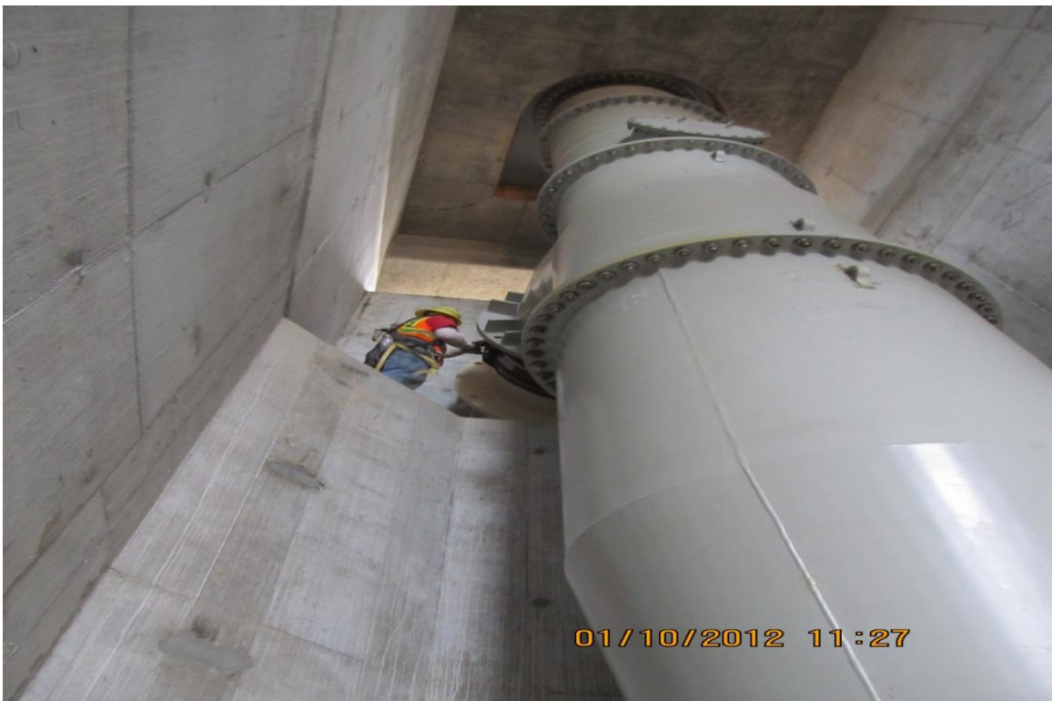
Balfour Beatty carpenter connects the first of two 60" pumps at the Pumping Plant.
